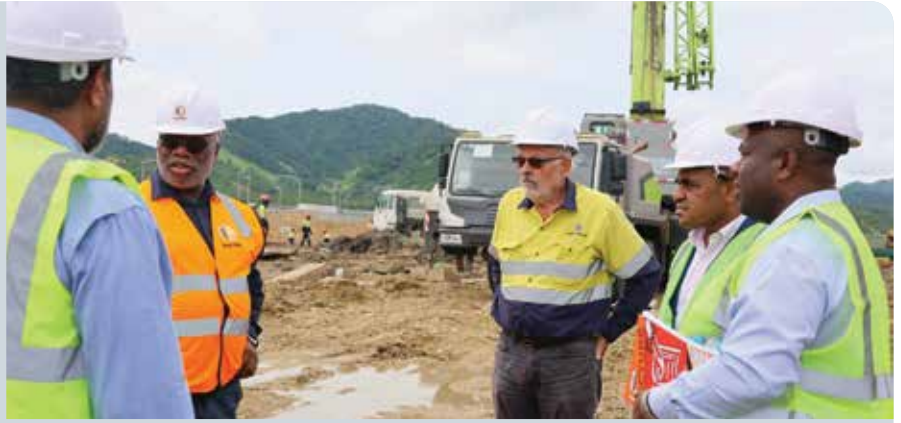
David Kavanamur, Managing Director of Kumul Consolidated Holdings (second from left) meets Wapu Sonk, Managing Director of KPHL (fourth from left) and his project management team at the new fuel storage facility being constructed at Motukea.
